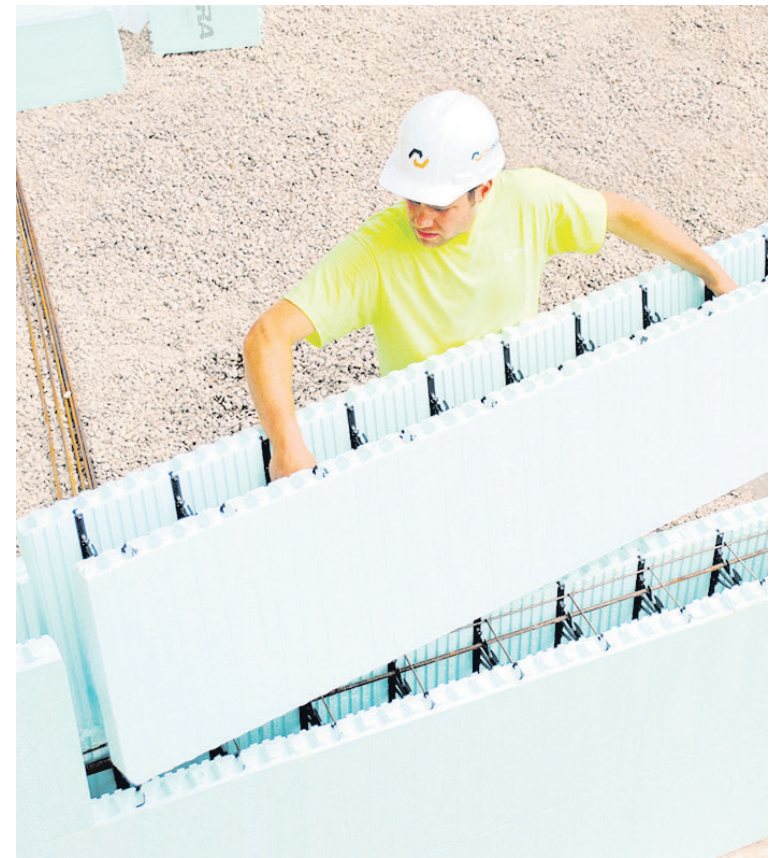
As building codes enforce tightened minimum standards for eco-responsibility, the more progressive builders are illustrating their own accountability by using and producing materials that are even more efficient than mandates demand.
